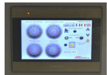
CONTROL PANEL BOARD WITH DISPLAY ON DHV LINE
